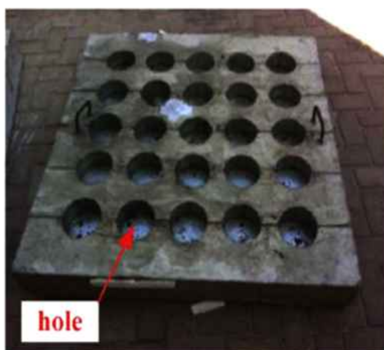
(c) Concrete roof with empty holes
